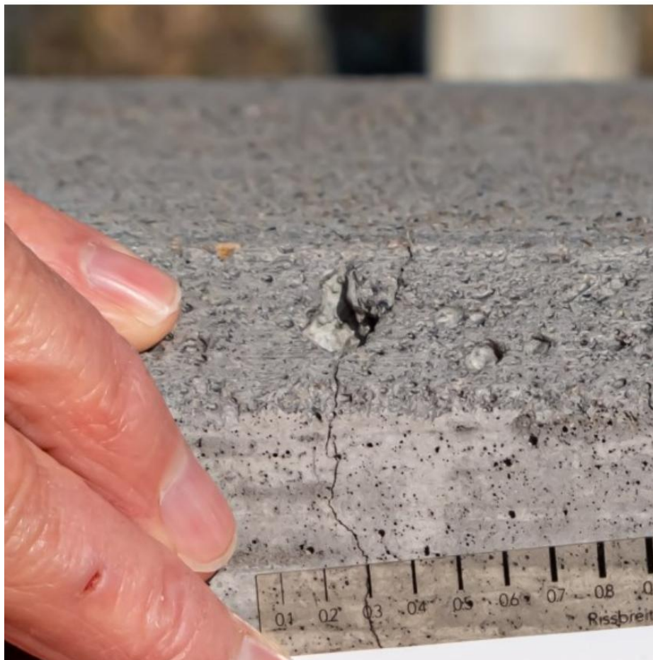
Parapet amont (sorte G), w \approx 0.3 \text{ mm}
